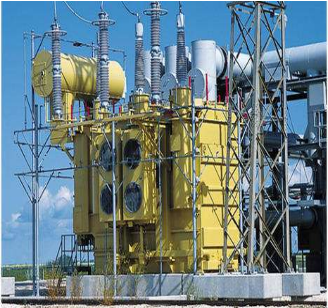
Figure 4.2: HVDC converter transformer
